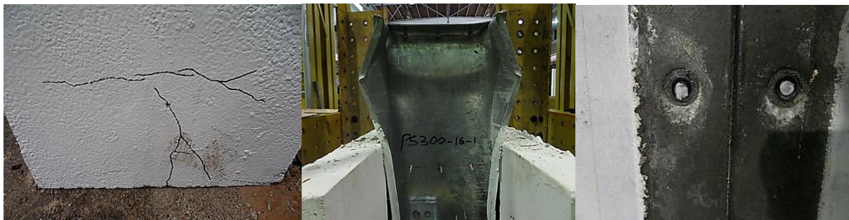
(a) Concrete Cracking and Crashing
