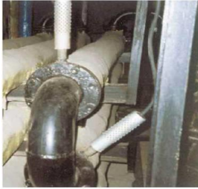
Fig. 1.1: Installation of Acoustics-T on a shell-and-tube water heater.
